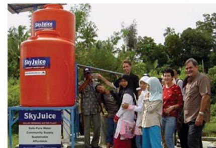
Water Treatment Plant in use at the Meulaboh school in December 2005.
